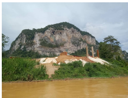
Gua Batu Kemirik , where developers levelled the land to create the site for the Sg. Nenggiri dam
