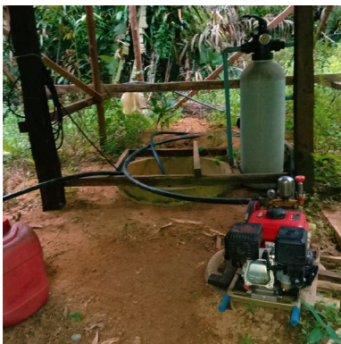
A photo of a ground-well pump used to source water
